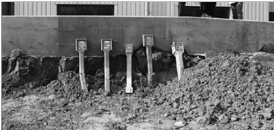
Subcontractors charged with building the car park removed pipeline markers from their original locations and placed them at the site's perimeter. Source: UK HSE (Fig. 4).
